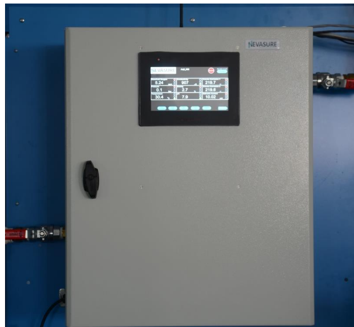
Figure 1: Hevasure Aquila-2s Monitoring Station
