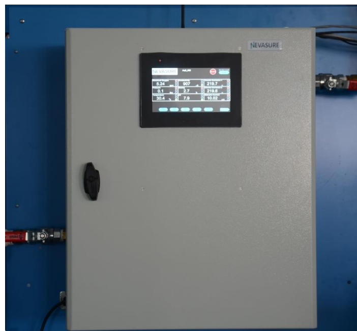
Figure 1: Hevasure Aquila-2+ Monitoring Station
